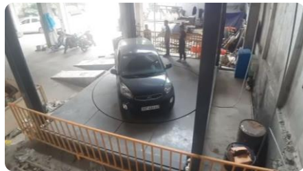
Turntable parking system
