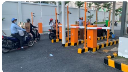
The controlling system
