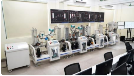
Distributed Control System
