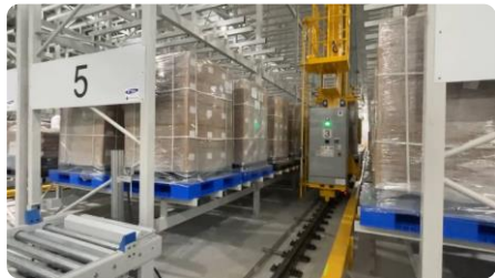
Automated storage and retrieval systems
